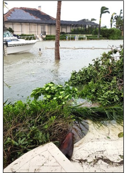
Water came within a foot of the step to my garage & house across to steps of lanai
