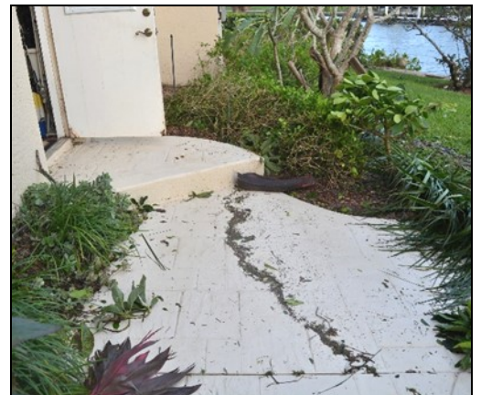
Residue leaves mark of water line just outside garage door
