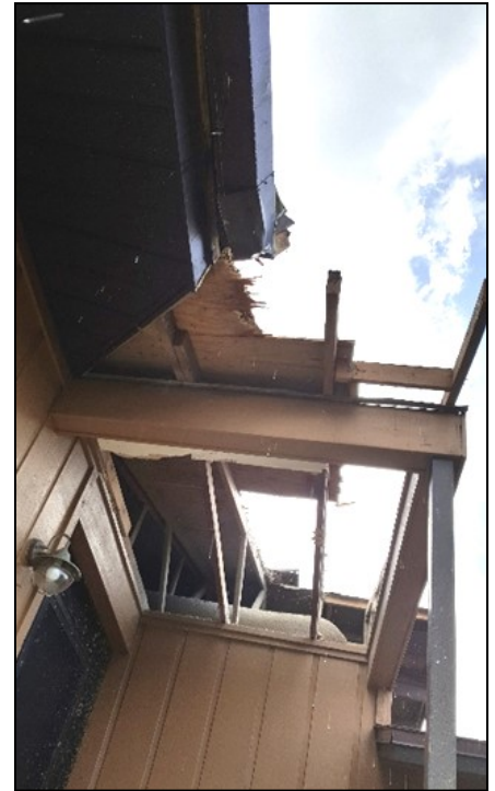
Partial loss of roof at Reiss' home
